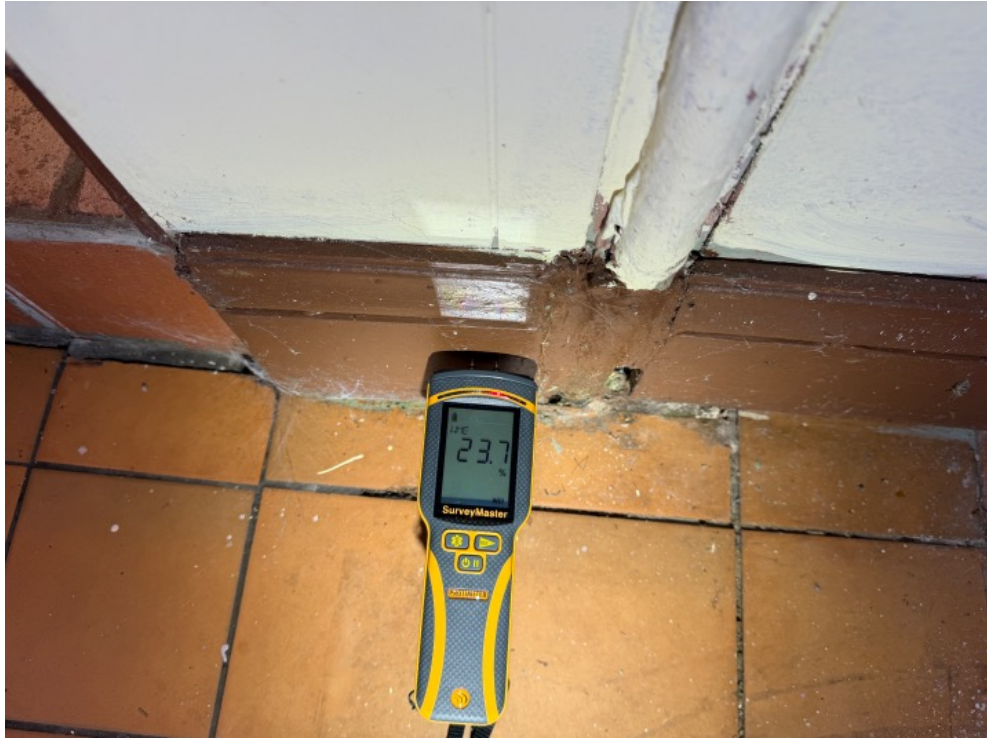
High moisture in utility room skirting boards
