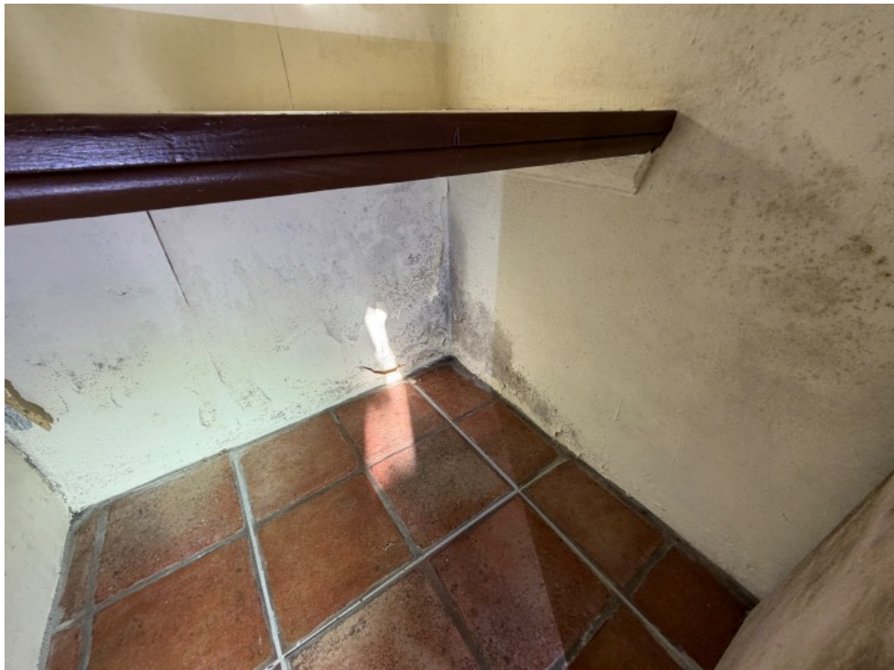
Black mould evidence in kitchen cupboard
