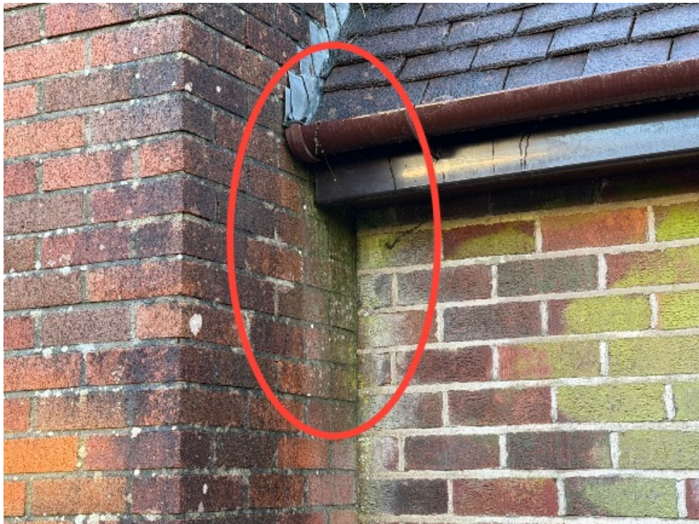
Staining observed beneath front gutter
