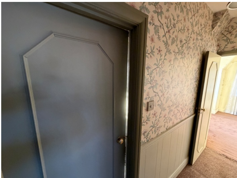
Bathroom door fouling in frame
