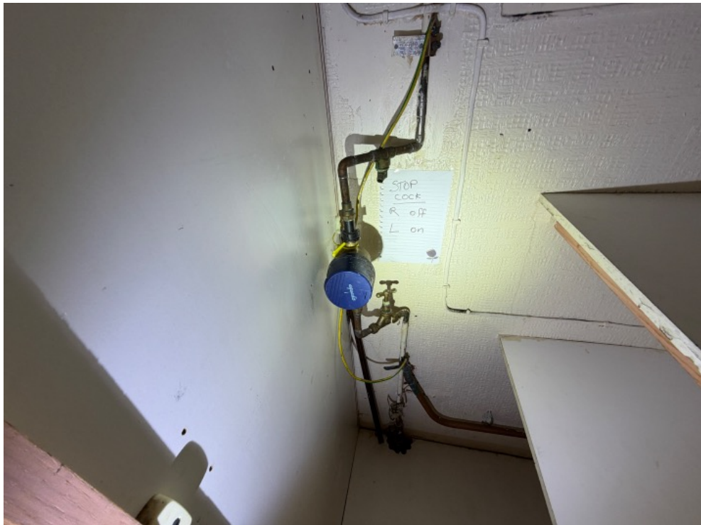
Incoming water main
