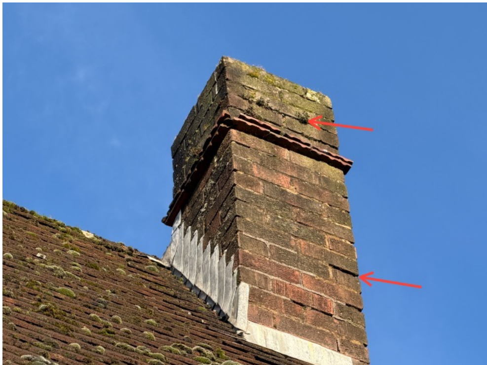
Left side chimney - vegetation and mortar missing
