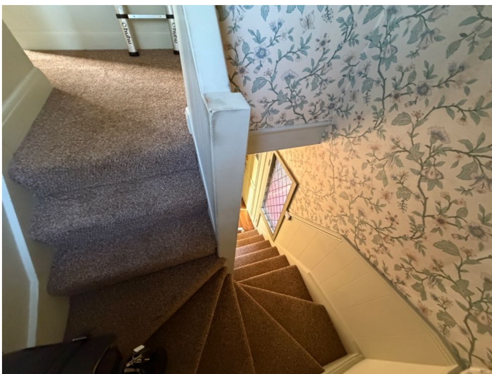
Lack of handrail to stairwell
