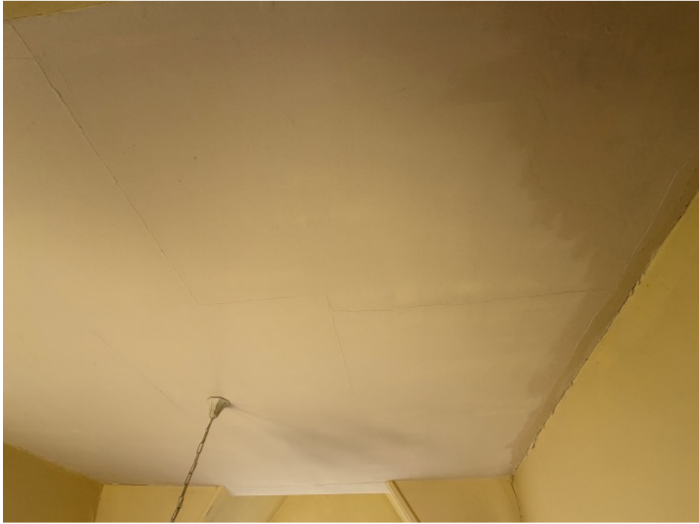
Hairline cracking to plasterboard junctions
