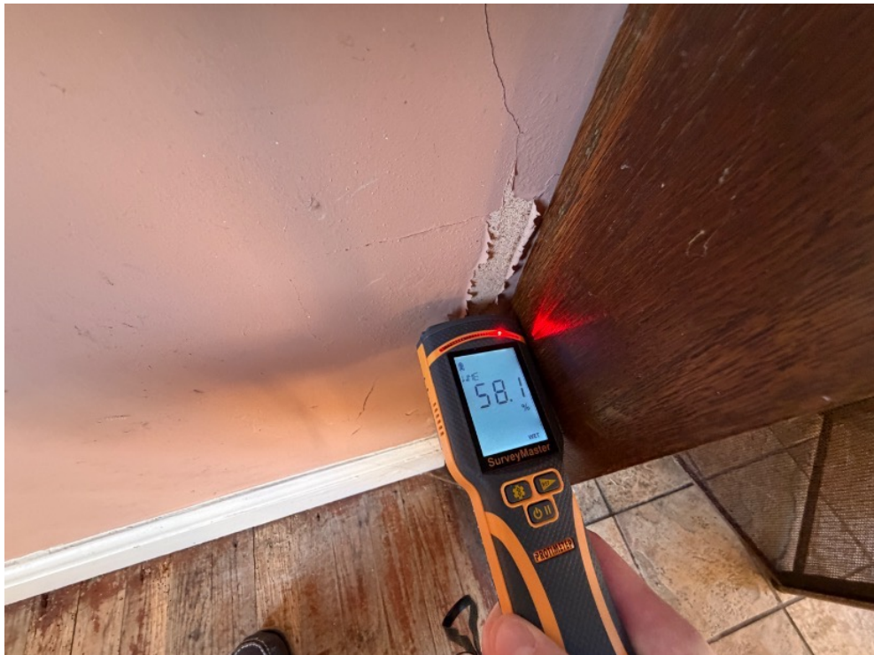
High moisture recorded in wall next to fireplace
