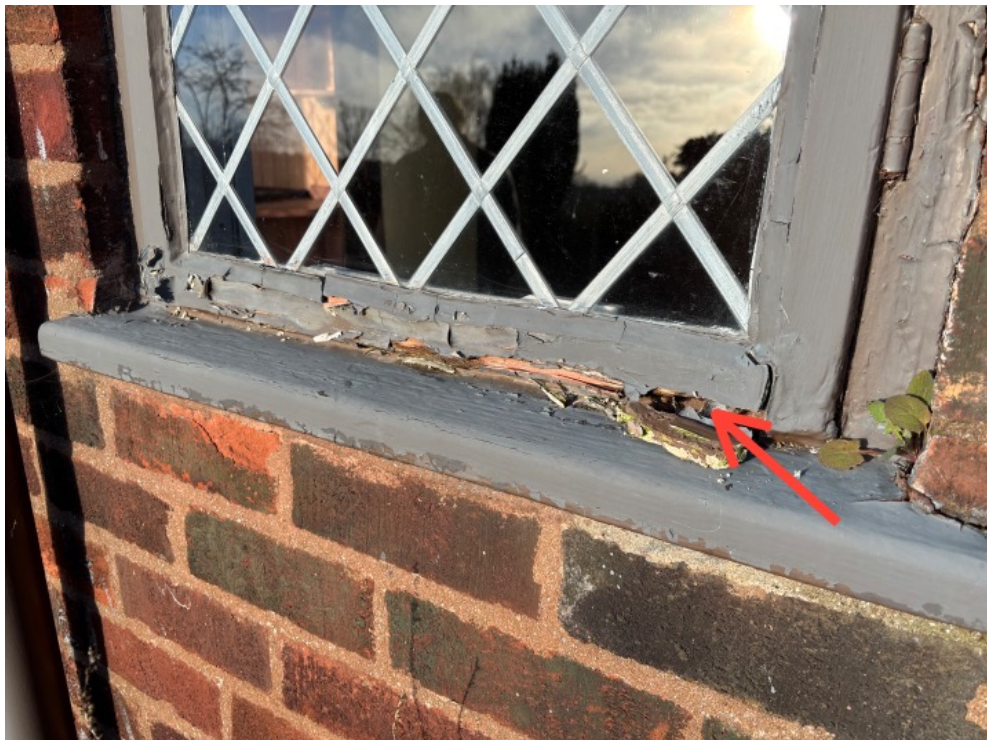
Decaying timber window frame
