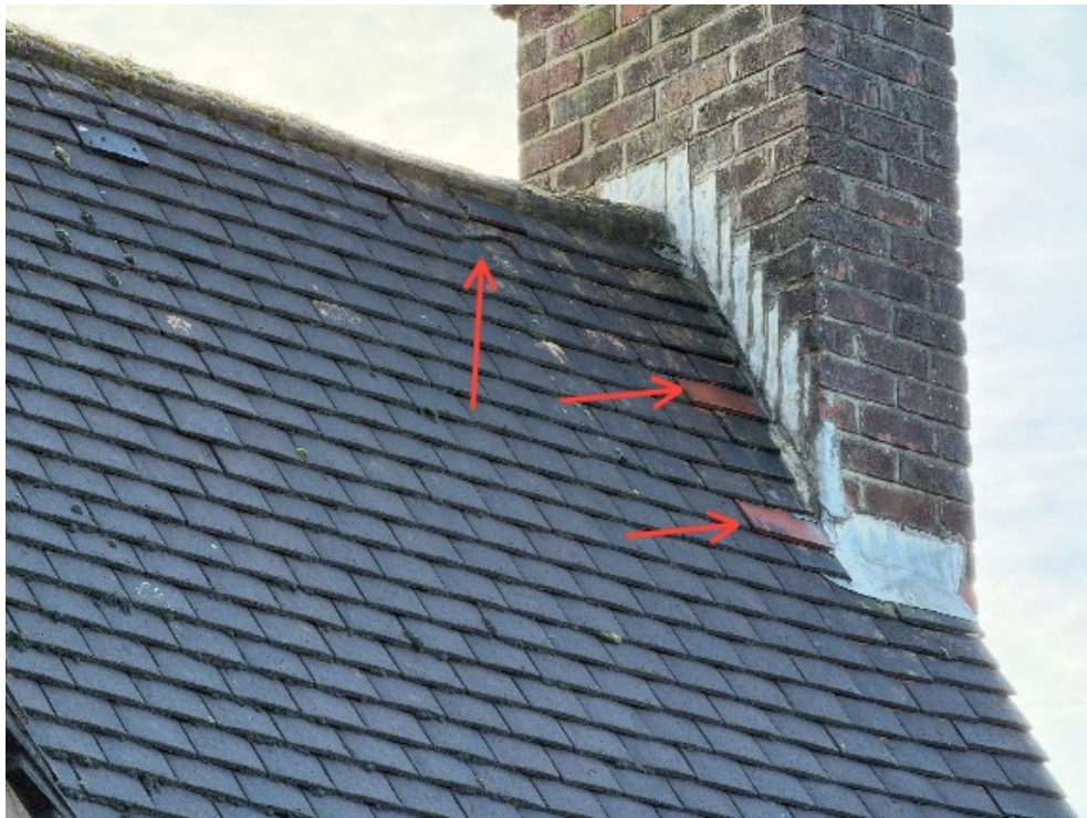
Damaged tile - roof repair sections
