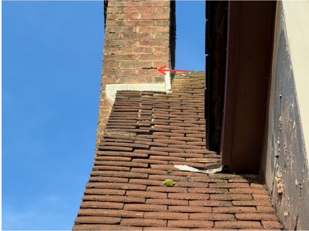
View of right side chimney - missing section of mortar
