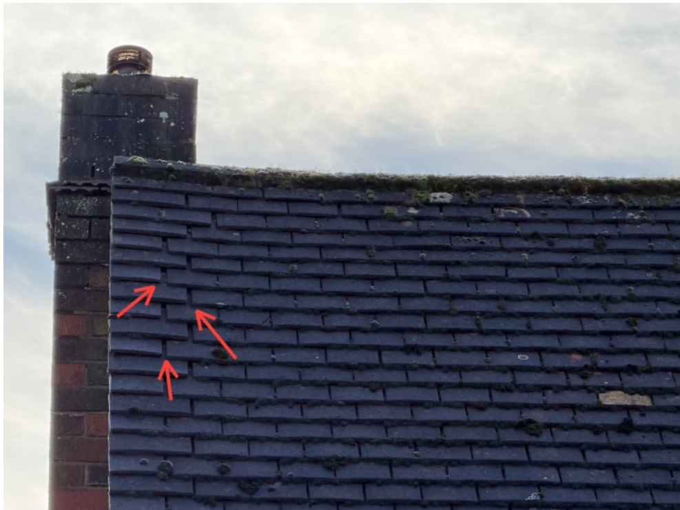
Wide spacing between tile joints
