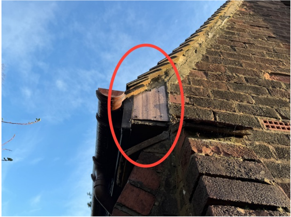
Missing end cap to right side external joinery
