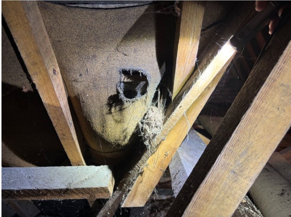
Evidence of nest behind roofing felt
