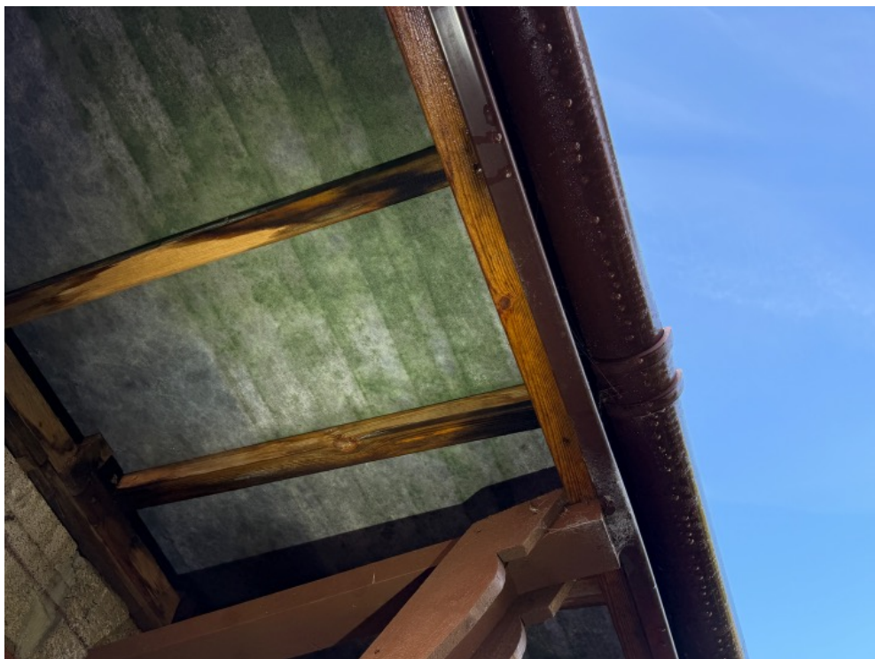
Water stained felt and roof timbers
