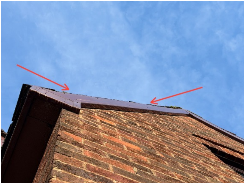
Lack of tile oversail to rear gable end bargeboard
