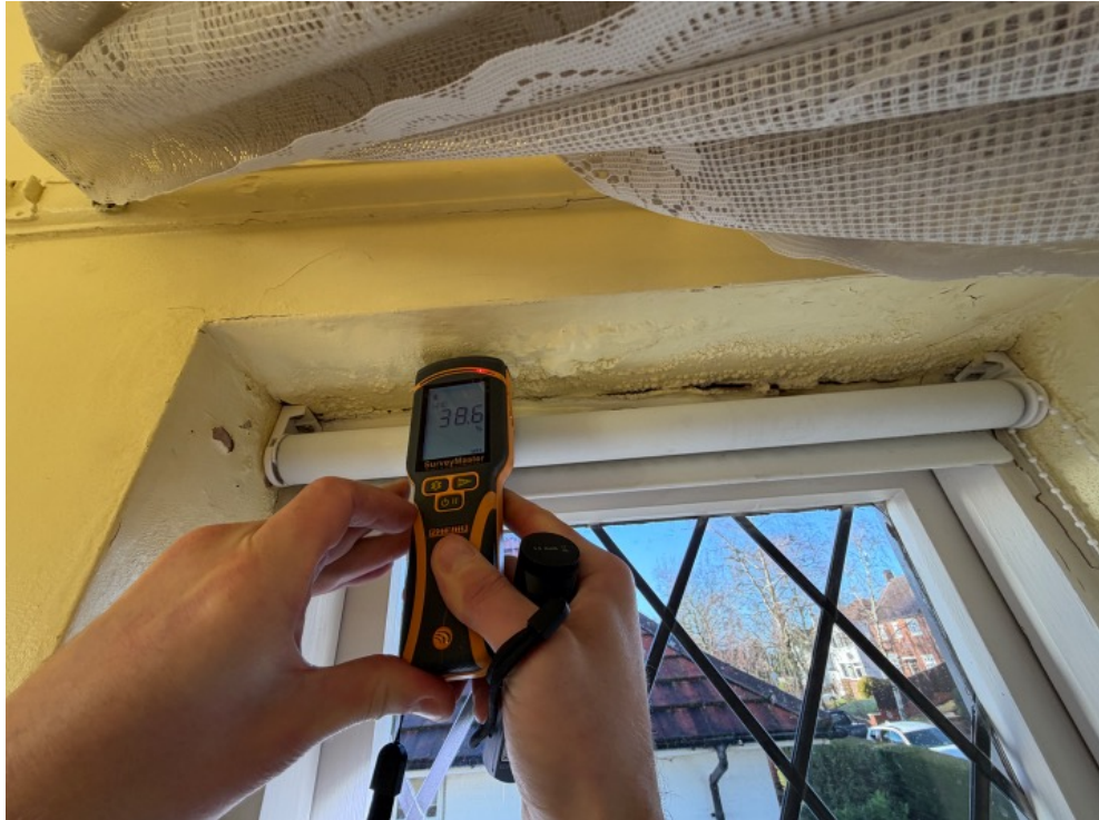
Dampness noted to bedroom 1 walls
