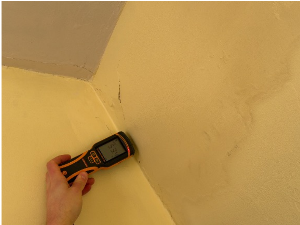
Dampness noted to ceiling in bedroom 1
