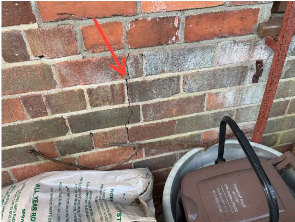
Fractured section of brickwork left side elevation
