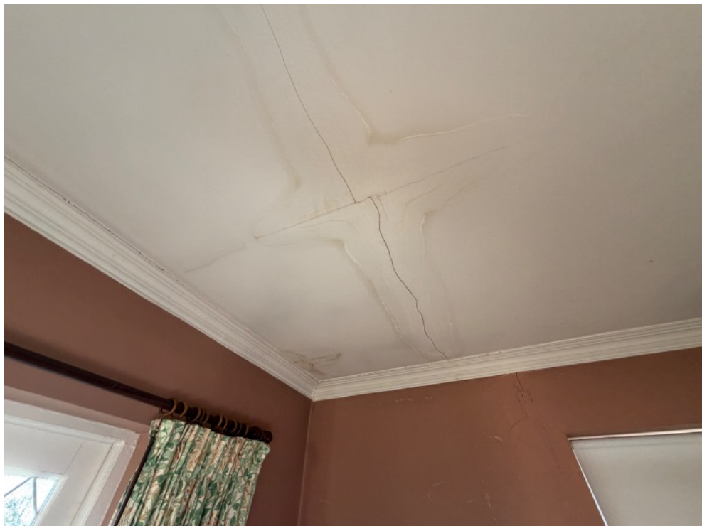
Moisture damaged ceiling - living room
