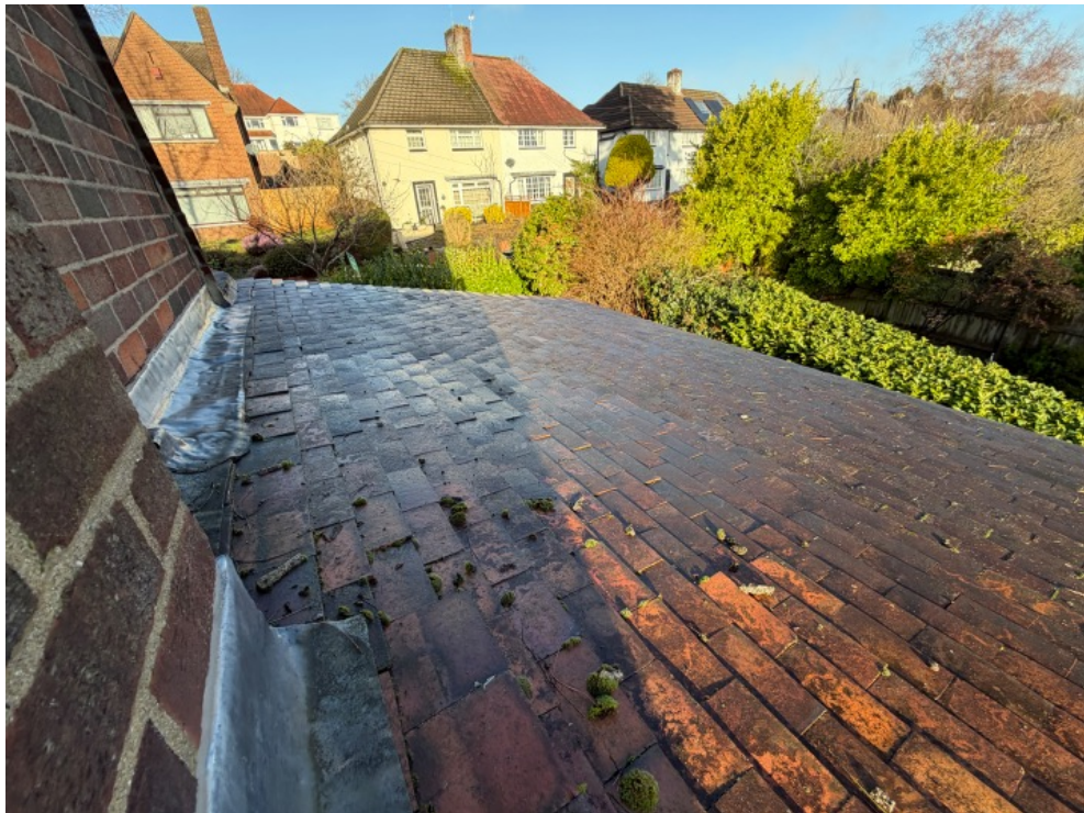
Lack of effective pitch to side roof
