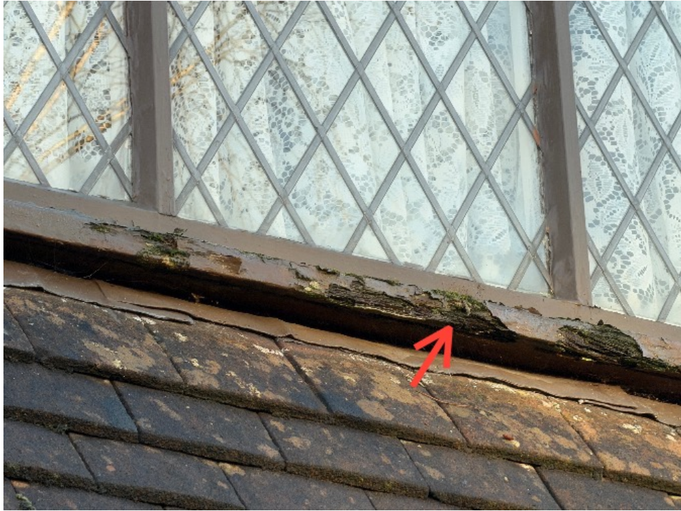
Decaying timber dormer window cill
