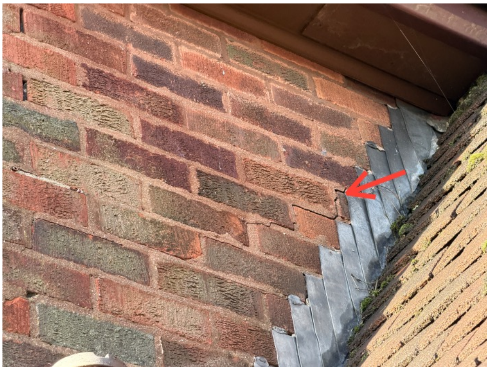
Hairline cracking to mortar joints
