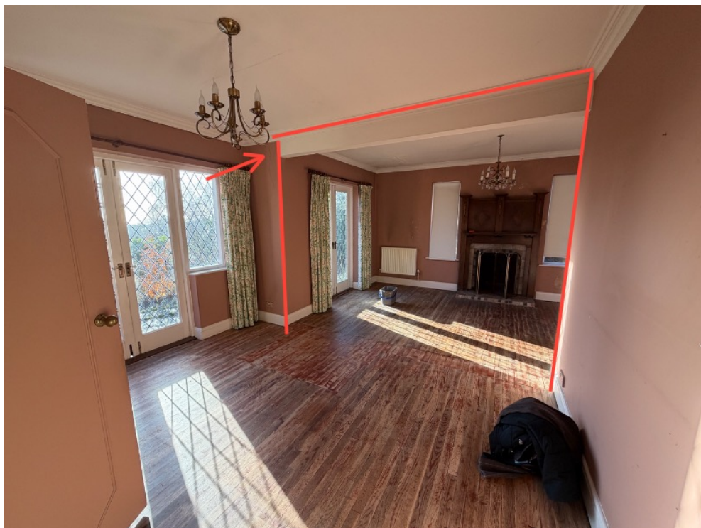
Wall removal from lounge - fracture in plaster
