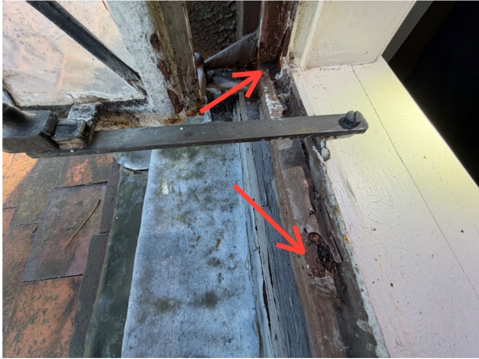
Corrosion to metal window frame
