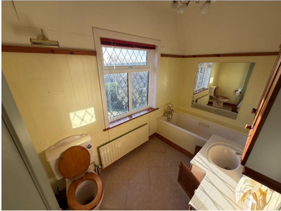
Lack of mechanical ventilation to bathroom
