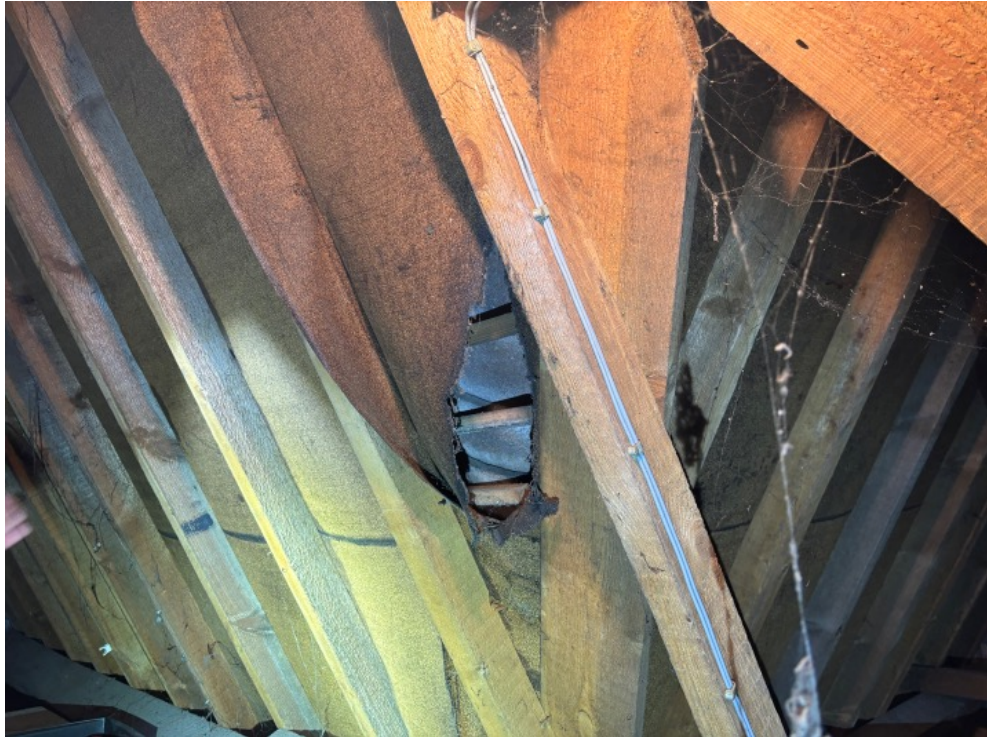
Torn roofing felt
