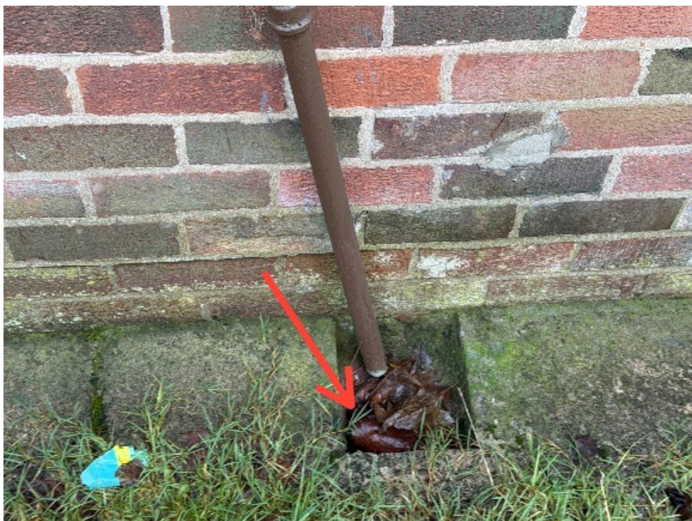
Detritus in gully
