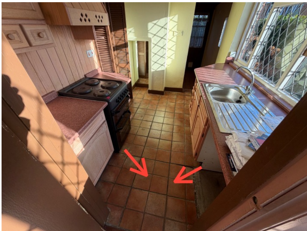
Uneven floor in kitchen
