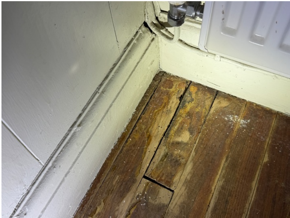
Moisture damaged and woodworm evidence to flooring in entrance hall beneath radiator valves
