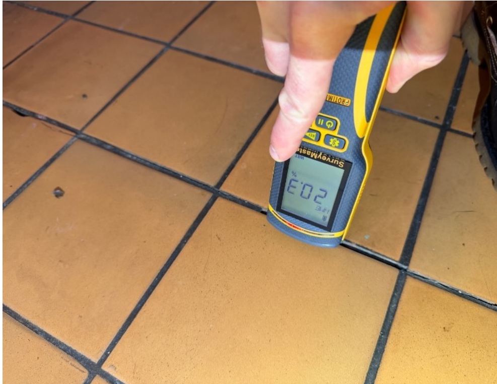
Moisture detected in utility room solid floor
