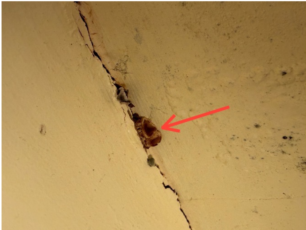
Fungal growth in bedroom 1
