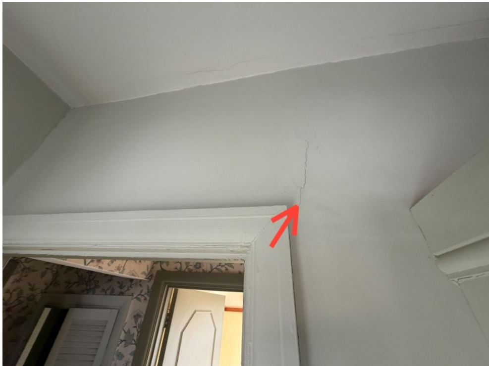
Hairline cracking above bedroom door
